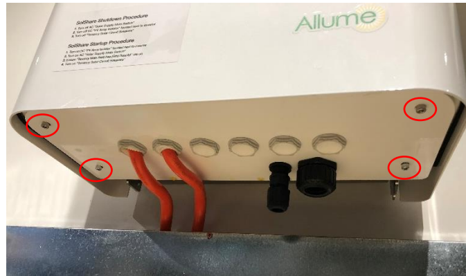
Fig 2. Opening SolShare installation Area
