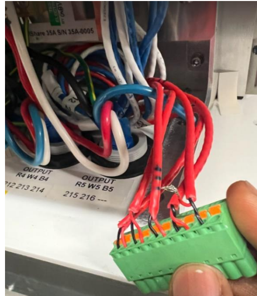
Fig 5. CT Block on red phase removed.
